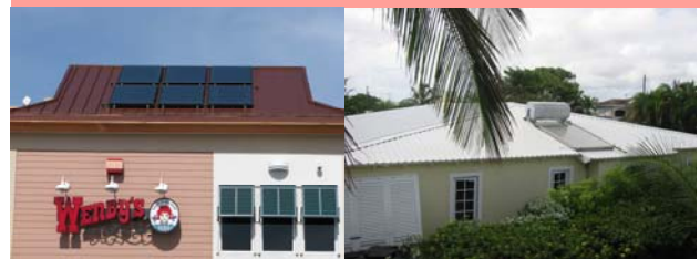
Flat plate solar water heater panels at Wendy's in Savannah, Grand Cayman (left), and an example of a batch collector system in Barbados (right)
