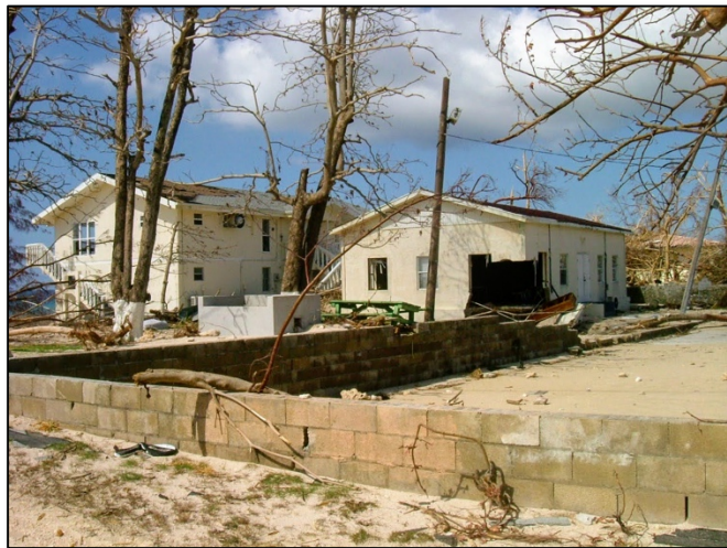
The Council office and the Prospect Youth Centre after Hurricane Ivan, September 2004.
