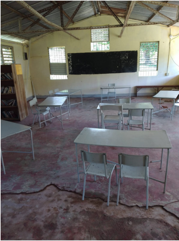
The interior in disrepair.
